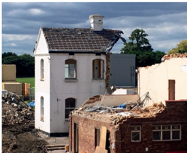
11 ▼ Part of the Jubilee Block, and the White House, during the 2018 demolition
